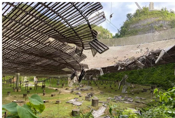
Damage caused by the failure of the first auxiliary cable in August | Image: UCF
